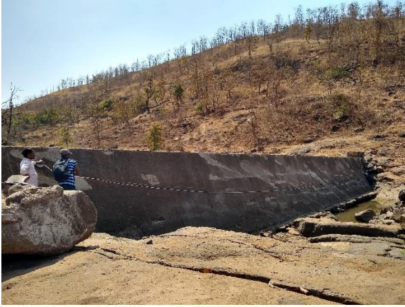
Figure 12: Damaged condition of CNB
