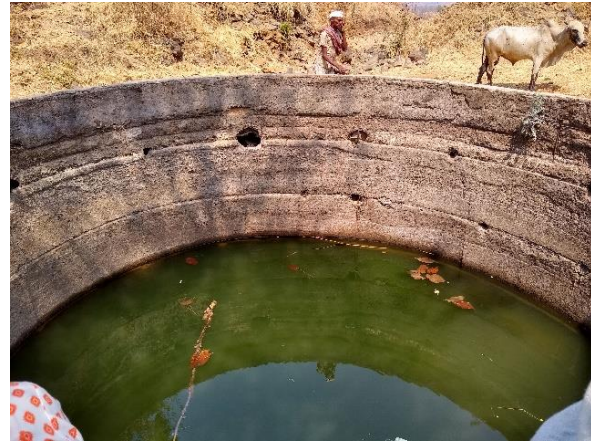
Figure 5: Depleted condition of Parapet wall, Waterproofing layer, Platform of PDW4 well
