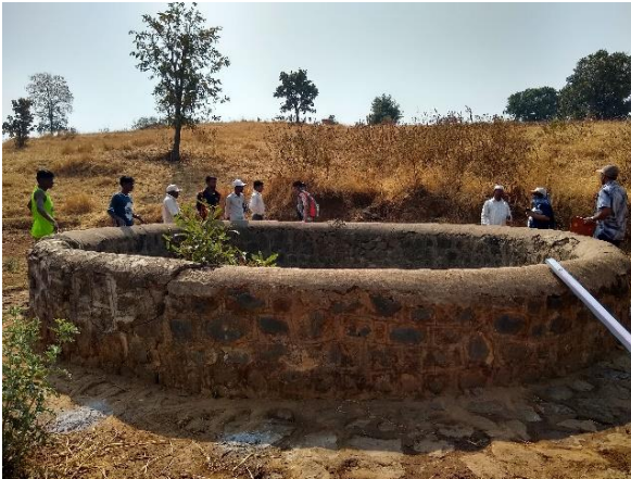
Figure 4: Partial damage in PDW1 well parapet wall
