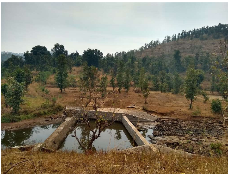
Figure 25: Water levels and condition of Aroehan Bund`
