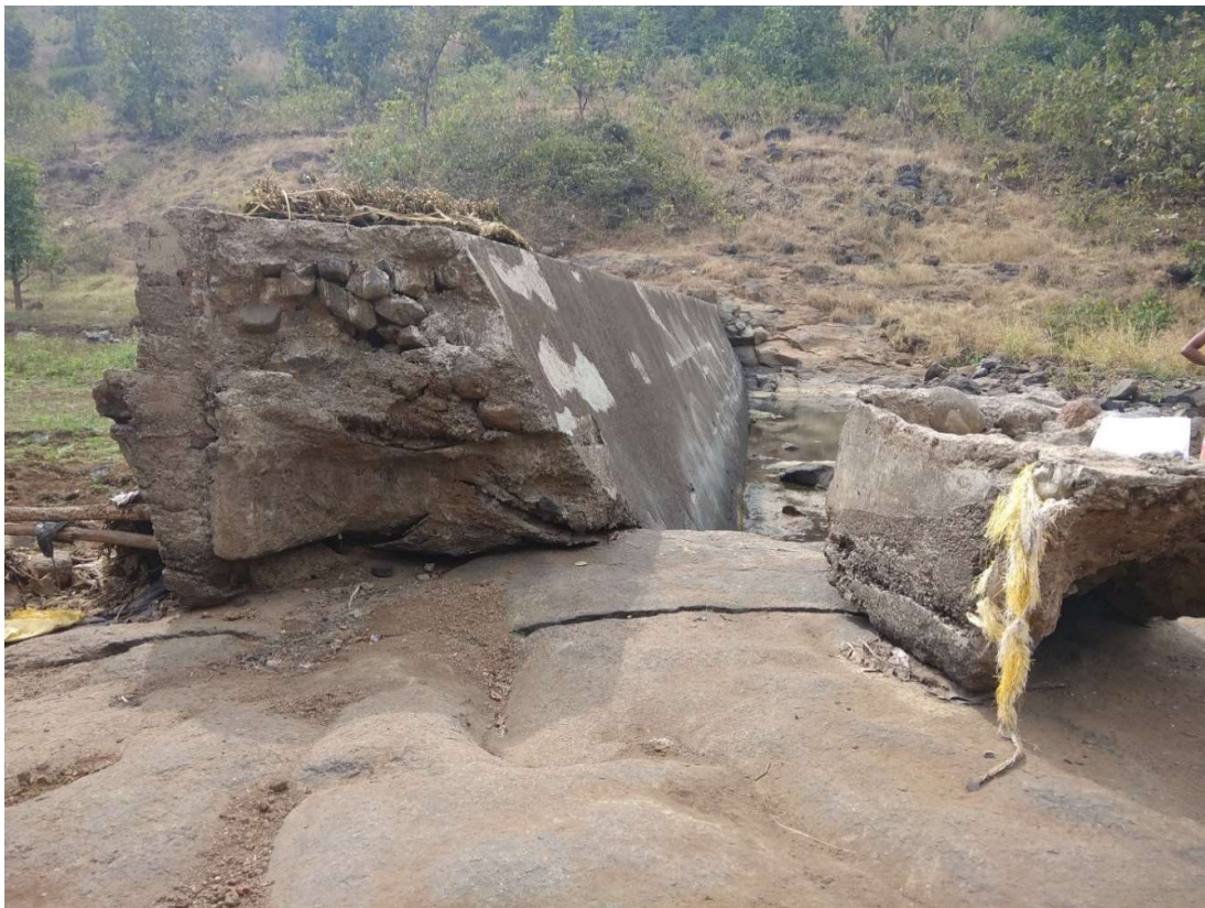
Figure 24: Fragmented condition of Government bund 1
